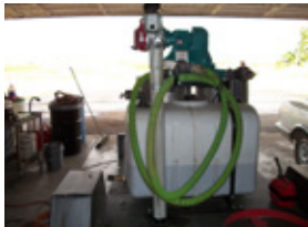
Waste oil skid mounted pump
