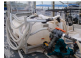
Pump out vessel
