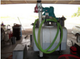
Waste oil skid mounted pump
