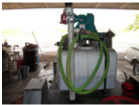
Waste oil skid mounted pump
