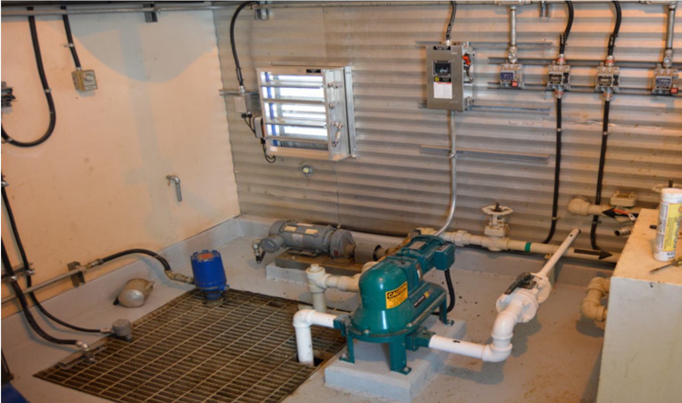
Mud Sucker 2FAC-EC installed at a wastewater pump house. Sump application. Pump transfers up to 20 GPM of wastewater and light solids. Shown with a three phase Siemens electric motor and SEW Eurodrive gear box. Other drive systems available.
