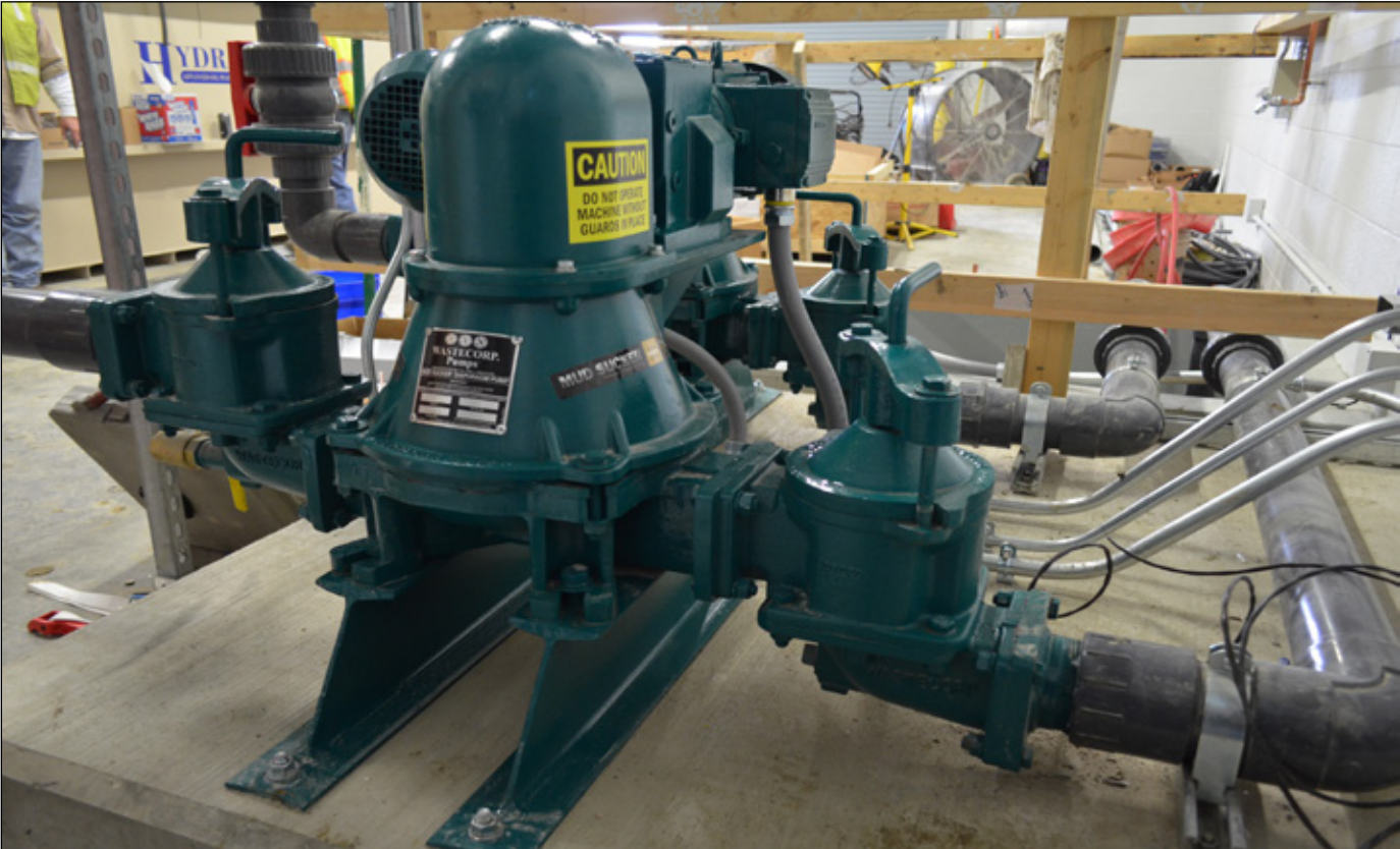
Mud Sucker B Series at a food processing facility. This application involves separating oil and waste water and then pumping for further treatment.
