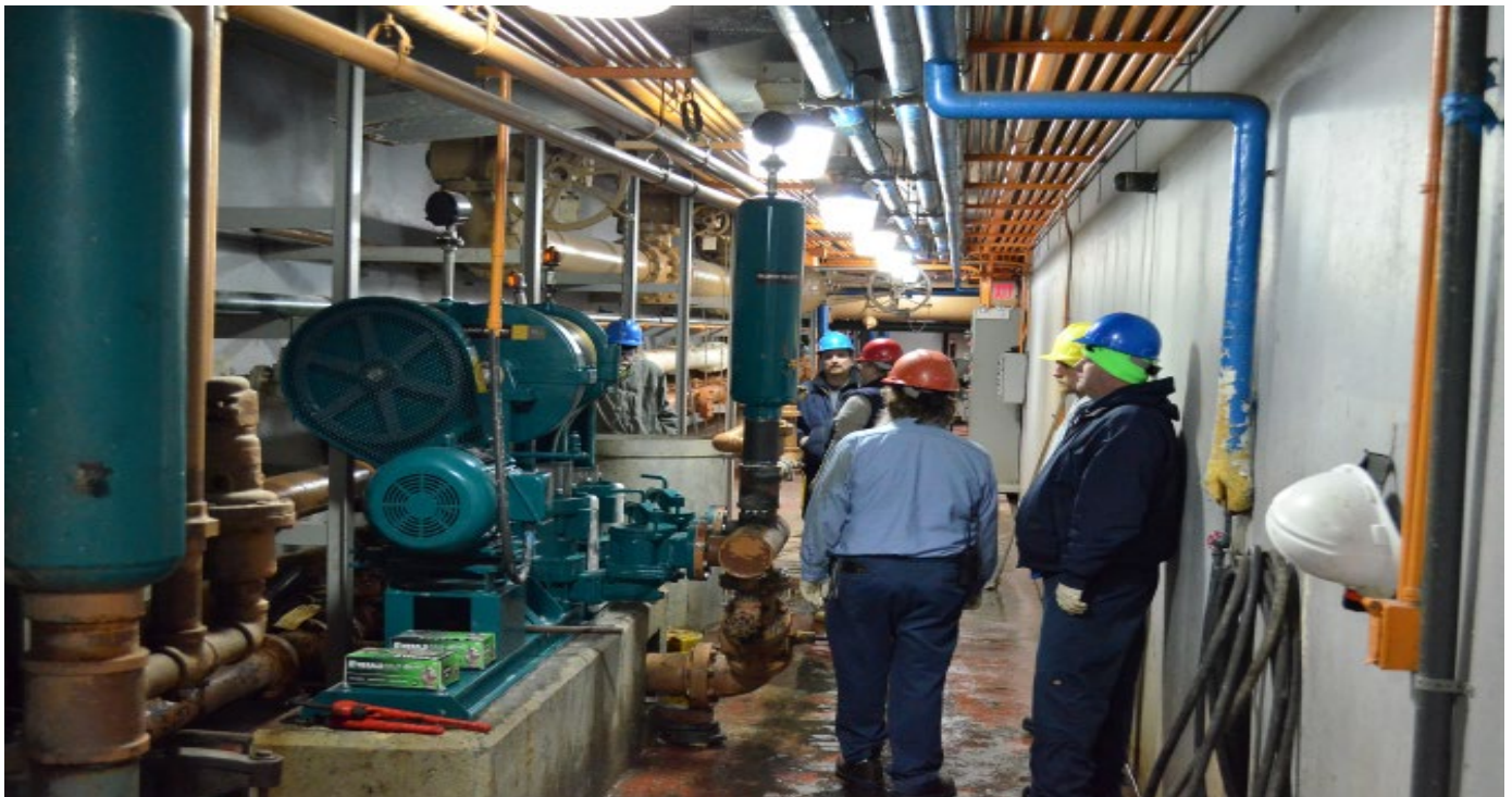
HPE 81W at a New Jersey wastewater treatment plant. The belt driven model has been favored by this facility's operators for decades. When it was time to replace the existing plunger pump the operators opted for the same belt driven design for enhanced pumping productivity.
