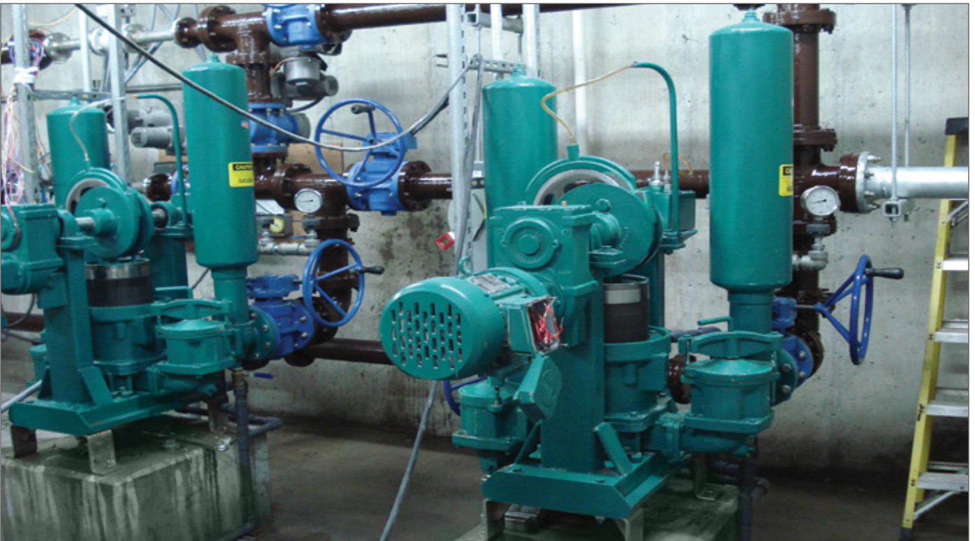
This Space Saver in Washington State replaced an existing double disc pump installation. No piping changes were needed because the pump configuration is similar.
