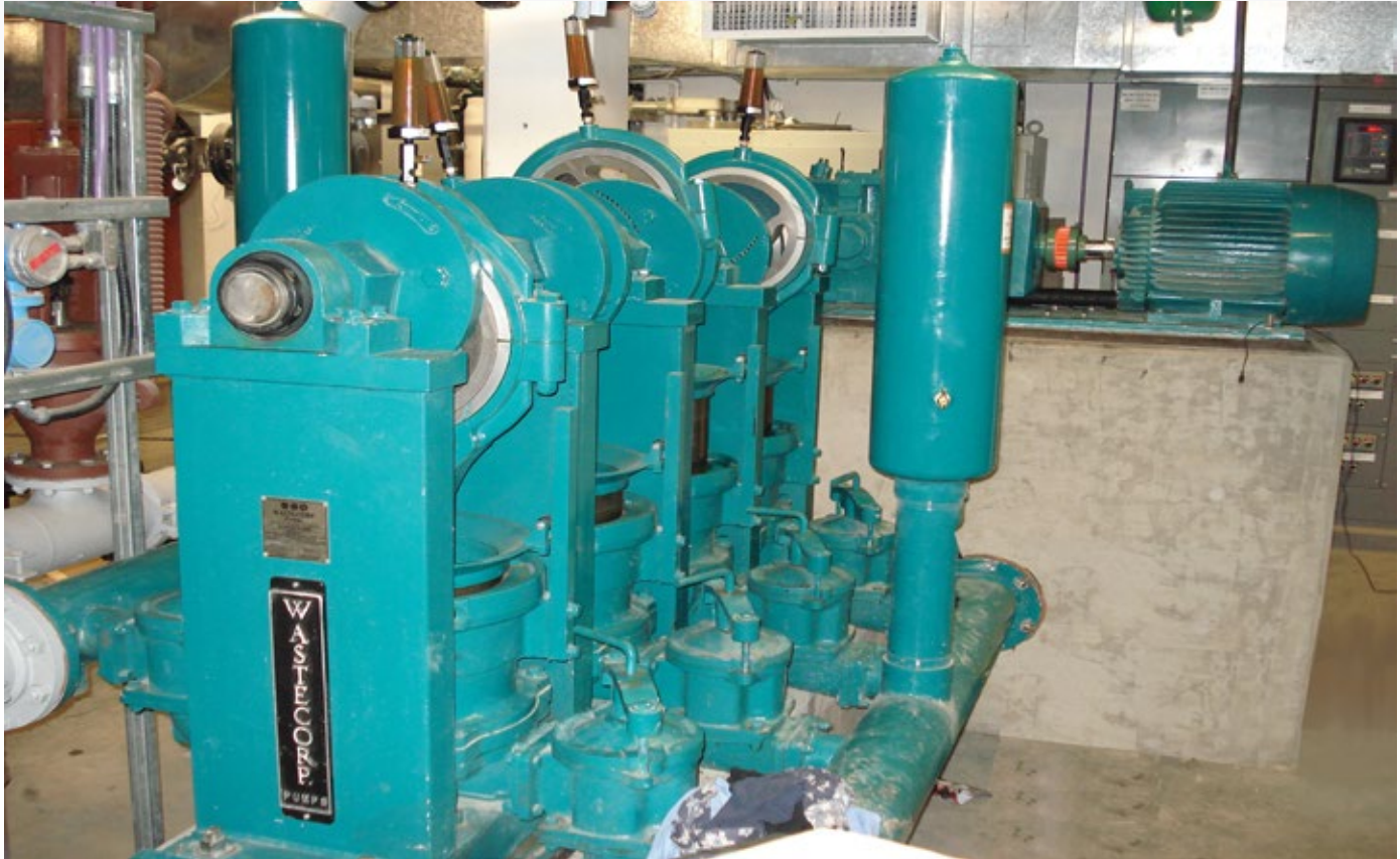
Wastecorp EHPE Series installed at a City of Edmonton, Alberta Canada wastewater treatment facility. Wastecorp installed eight plunger pumps at the facility as part of a multi-year upgrade/expansion.
