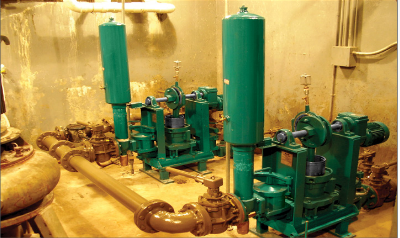
Space Saver's transferring sewage at a Knoxville, Tennessee sanitary district plant. With no base requirements, your Space Saver plunger pump options are almost endless.
