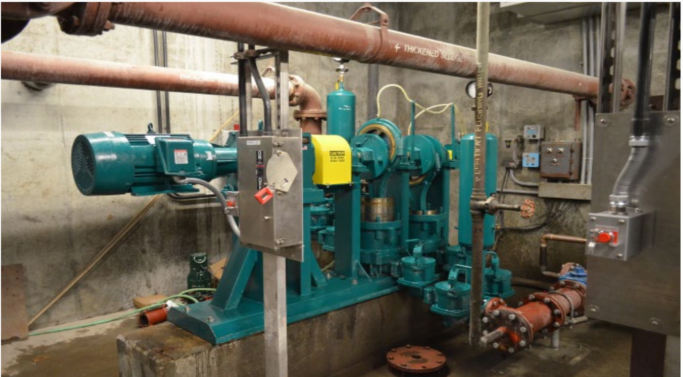
HPE-1142 plunger pump at a Boston, MA water pollution control facility. Pump includes a direct drive motor with a block heater to manage seasonal changes in weather. Higher head application which included dual ball valves for thicker slurry and sludge.
