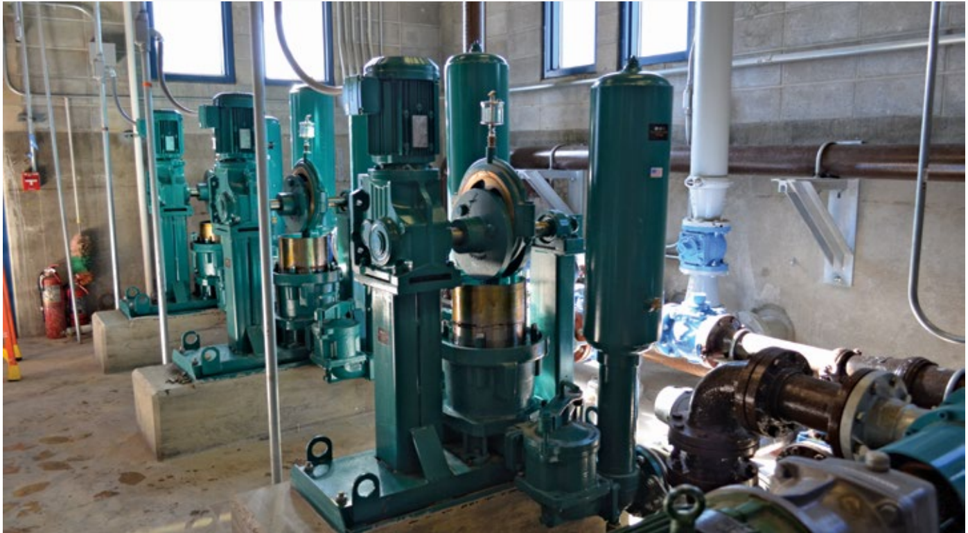
Model PE-9-SS Plunger pump in a Riverside County, California wastewater treatment plant. The facility replaced rotary lobe pumps with next generation plunger pump technology. The space saving design shown reduces the pump footprint by 35%. Application involves pumping thickened fermented sludge from a digester.
