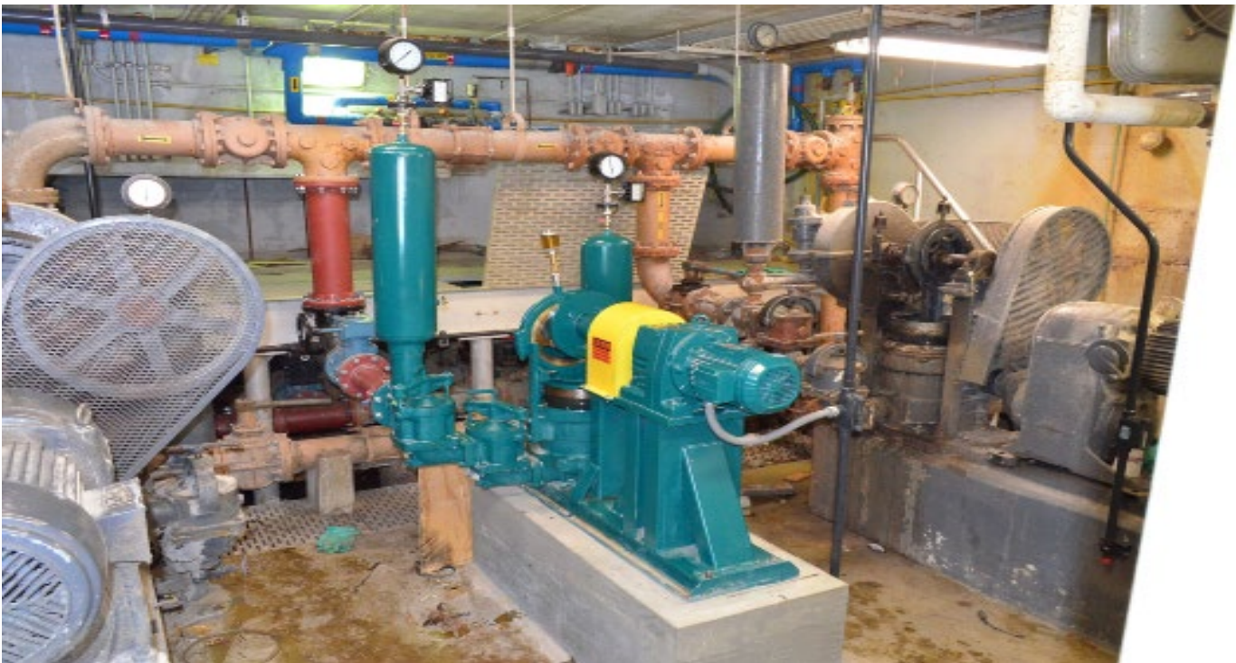
Model PE-941 dual ball valve at an upstate New York municipal sewage treatment facility. Facility upgrade involved upgrading control panels and pumping equipment. Wastecorp replaced Koline Sanderson and Carter plunger pumps. Dual ball valve configuration assists in pumping high solids above 15%.
