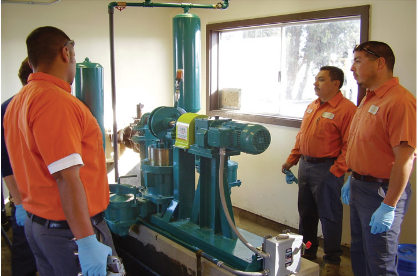
Wastecorp PE 941 plunger installation at a northern California wastewater treatment plant. Wastecorp offers start-up and staff training services from the factory or our worldwide dealer network.
