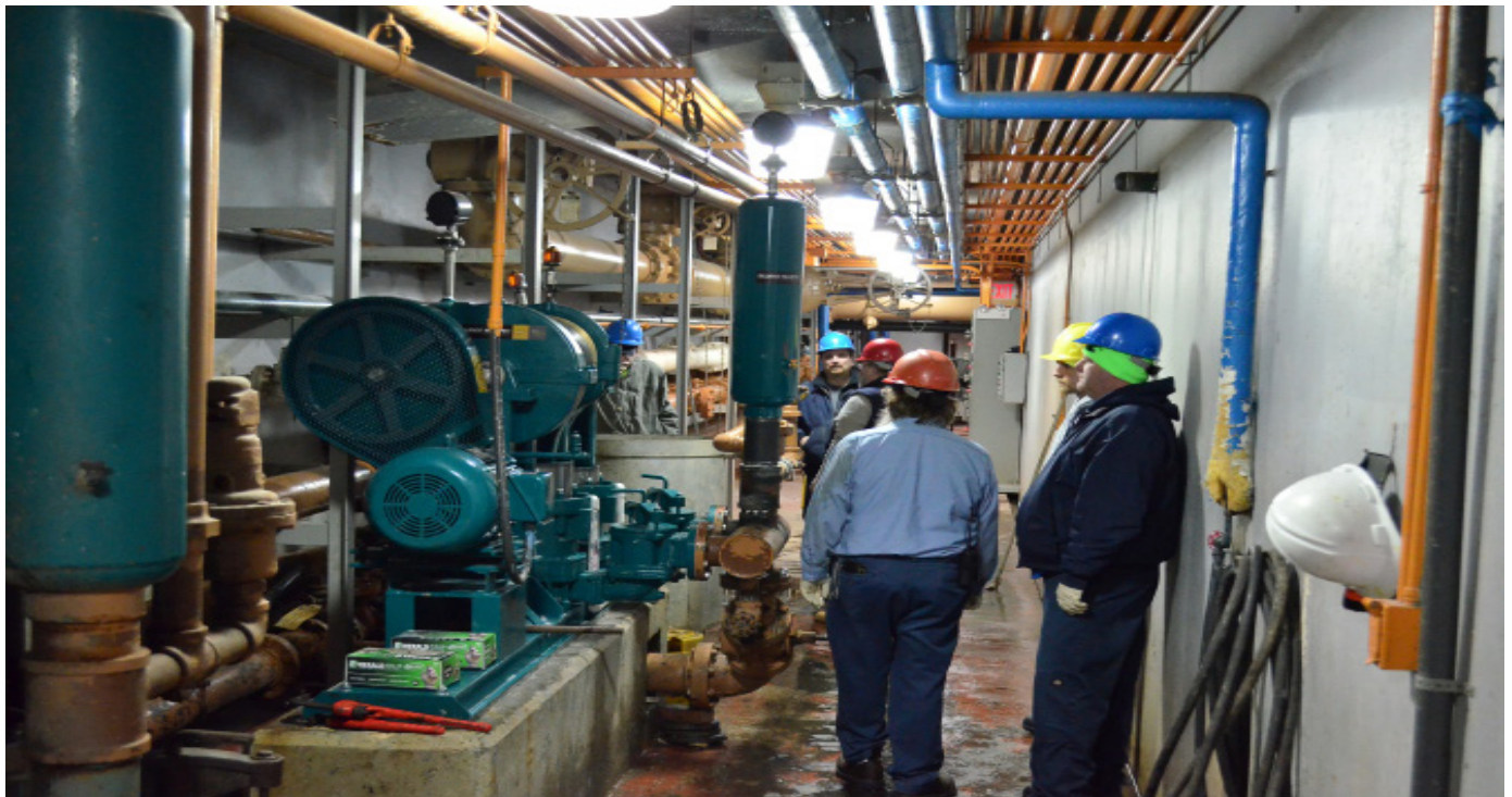
HPE 81W at a New Jersey wastewater treatment plant. The belt driven model has been favored by this facility's operators for decades. When it was time to replace the existing plunger pump the operators opted for the same belt driven design for enhanced pumping productivity.
