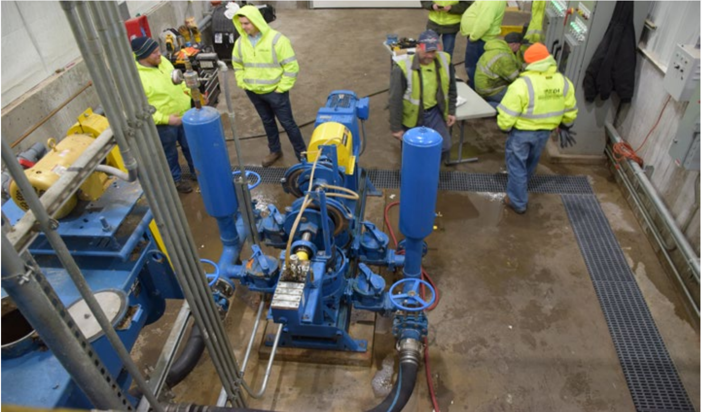
Wastecorp HPE 1142 plunger pump at an upstate New York sewage treatment facility. This facility has used plunger pumps for their primary sewage process for over 40 years. This new pump is a direct replacement.
