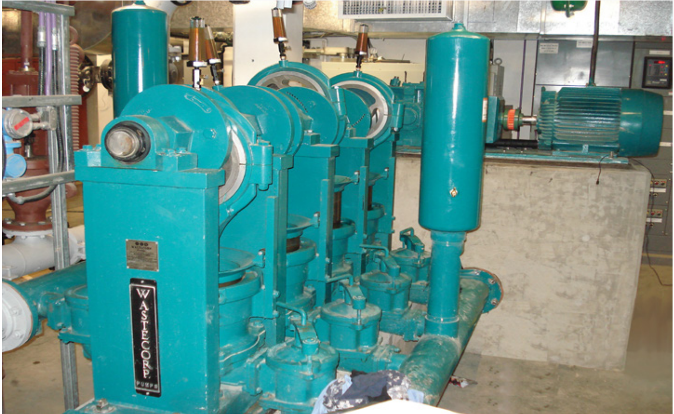
Wastecorp EHPE Series installed at a City of Edmonton, Alberta Canada wastewater treatment facility. Wastecorp installed eight plunger pumps at the facility as part of a multi-year upgrade/expansion.
