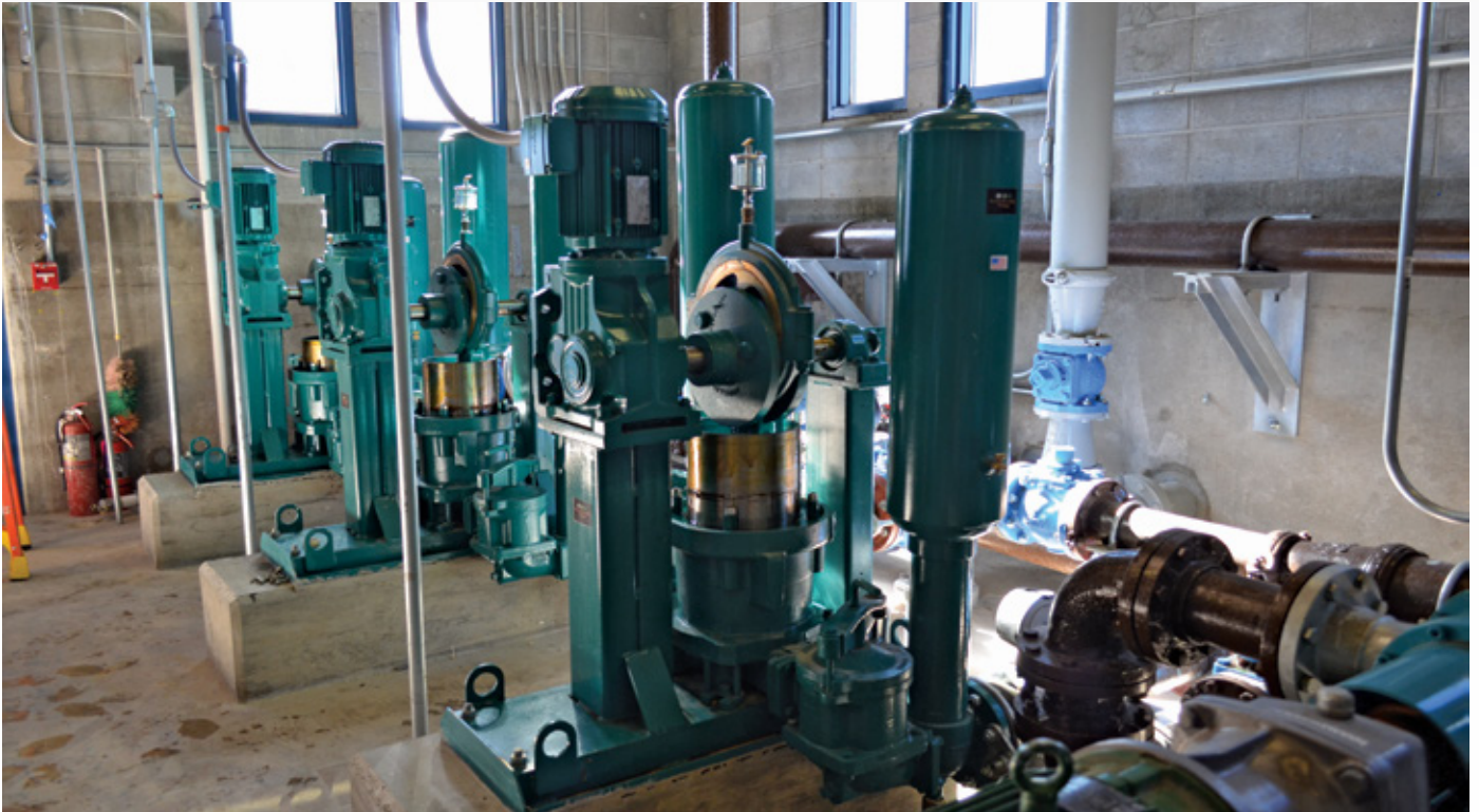
Model PE-9-SS Plunger pump in a Riverside County, California wastewater treatment plant. The facility replaced rotary lobe pumps with next generation plunger pump technology. The space saving design shown reduces the pump footprint by 35%. Application involves pumping thickened fermented sludge from a digester.
