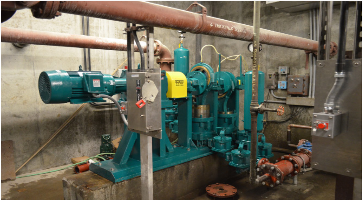
HPE-1142 plunger pump at a Boston, MA water pollution control facility. Pump includes a direct drive motor with a block heater to manage seasonal changes in weather. Higher head application which included dual ball valves for thicker slurry and sludge.
