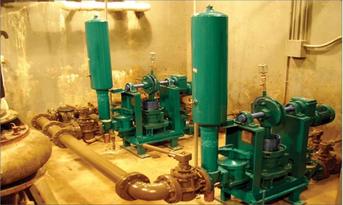
Space Saver's transferring sewage at a Knoxville, Tennessee sanitary district plant. With no base requirements, your Space Saver plunger pump options are almost endless.
