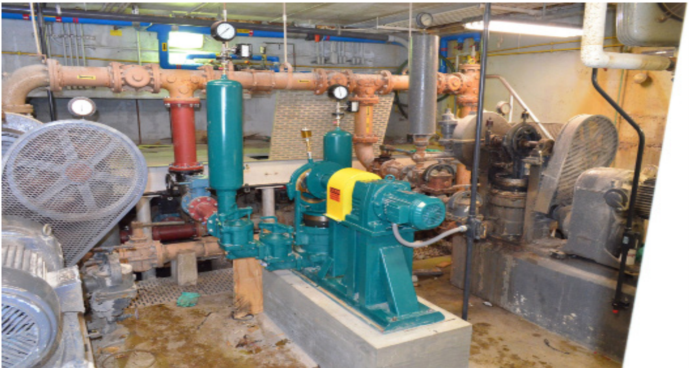
Model PE-941 dual ball valve at an upstate New York municipal sewage treatment facility. Facility upgrade involved upgrading control panels and pumping equipment. Wastecorp replaced Koline Sanderson and Carter plunger pumps. Dual ball valve configuration assists in pumping high solids above 15%.
