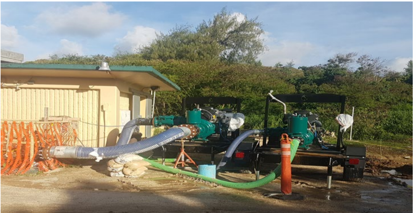
Trash Flow TFV-6 at a Miami, Florida food processing facility. The Trash Flow dry prime pumps help to prevent overflowing lagoons and storm sewers during the rainy season and during storms. Options include DOT compliant trailer packages with LOFA control panels and 50' of suction/discharge hose.
