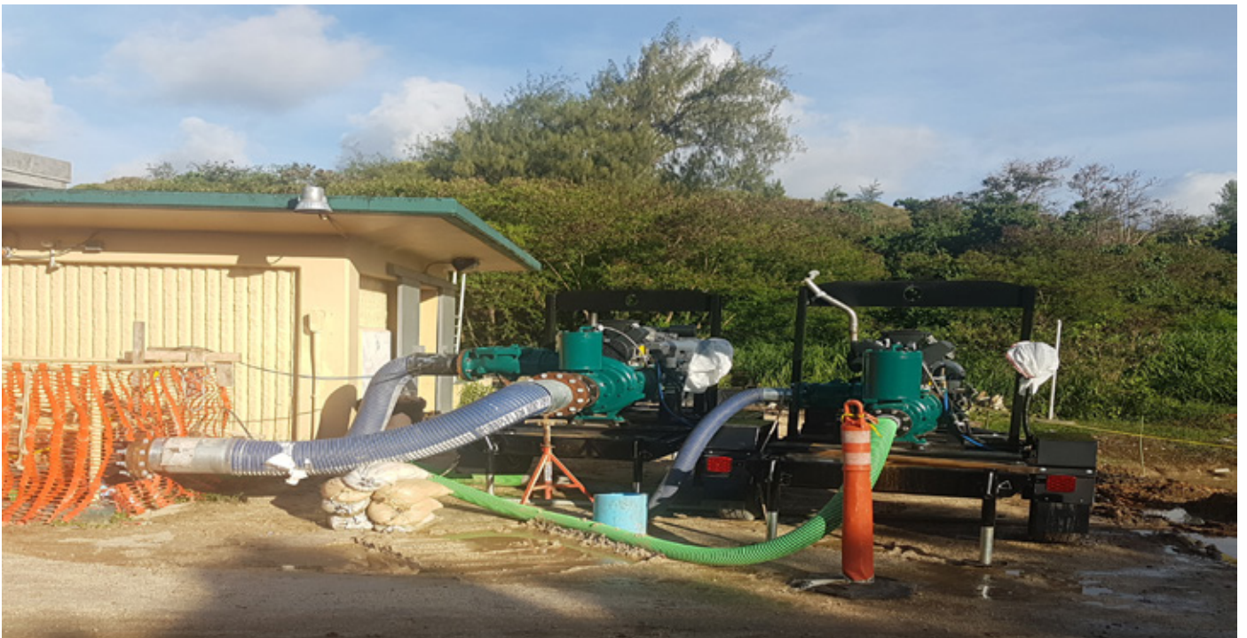
Trash Flow TFV-6 at a Miami, Florida food processing facility. The Trash Flow dry prime pumps help to prevent overflowing lagoons and storm sewers during the rainy season and during storms. Options include DOT compliant trailer packages with LOFA control panels and 50' of suction/discharge hose.
