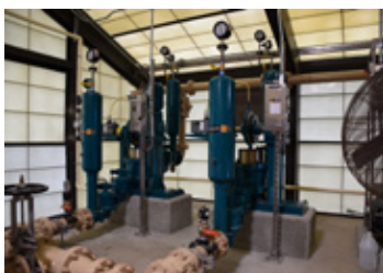
Space Saver Series replacing rotary lobe pumps at a WWTP
