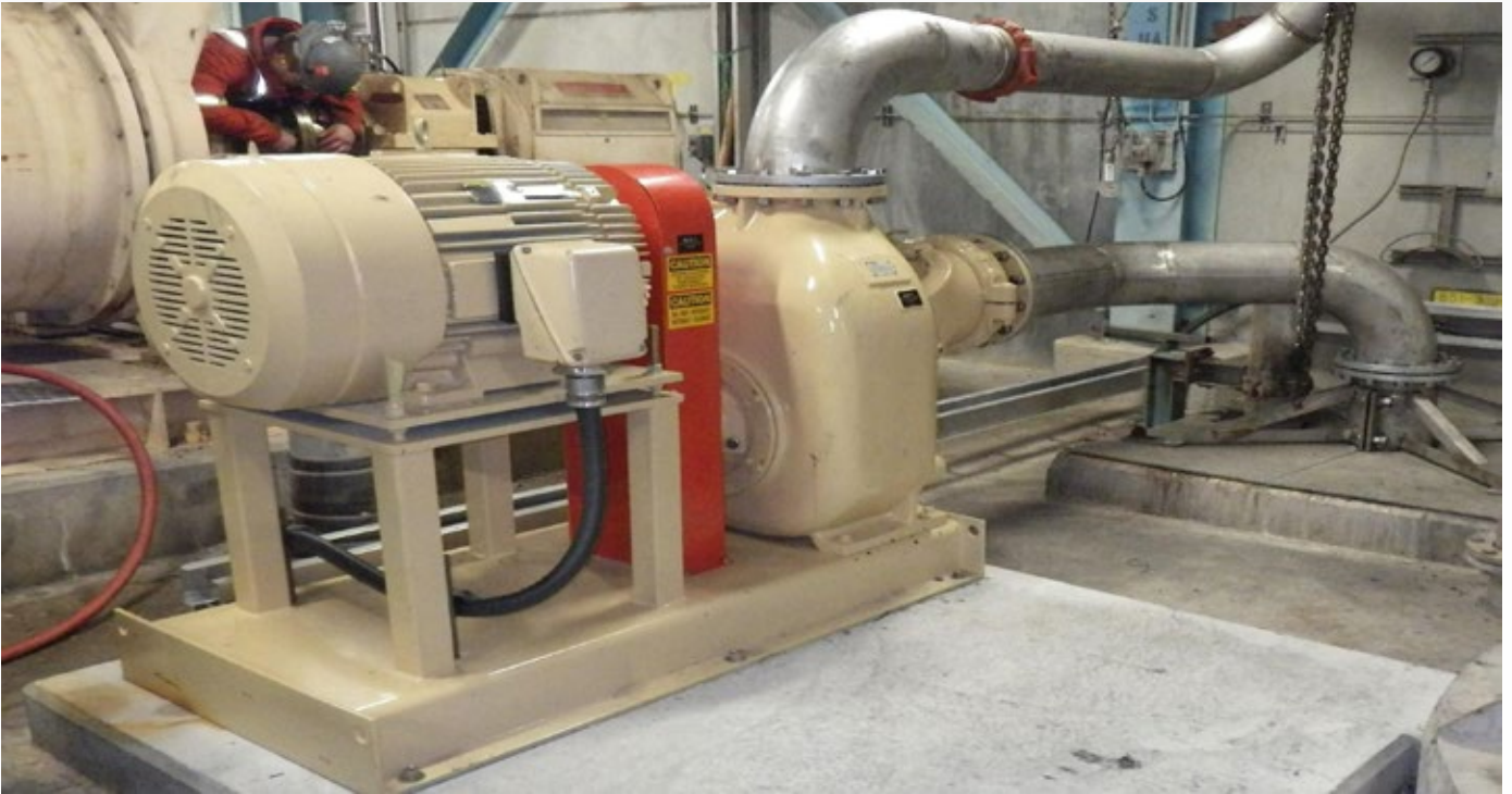
PULP AND PAPER TRANSFER PUMPS Shown TFCC-10 installed at a multinational paper mill in Wisconsin. Belt driven model shown.
