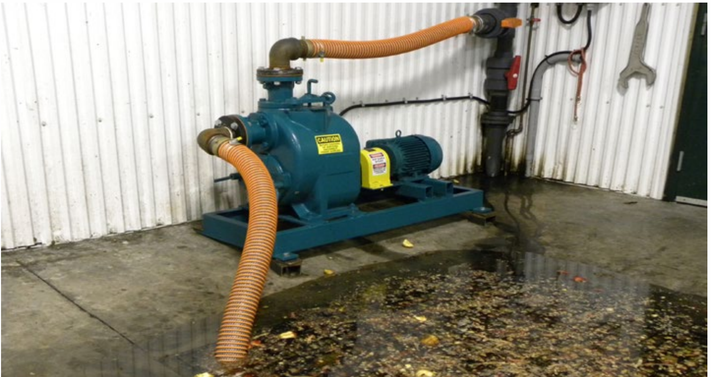
FOOD PROCESSING PUMPS Shown Trash Flow TFCC-3 installed at a Massachusetts food processing facility. End user pumps apple cores, skins and other solids. Close coupled direct drive model shown.
