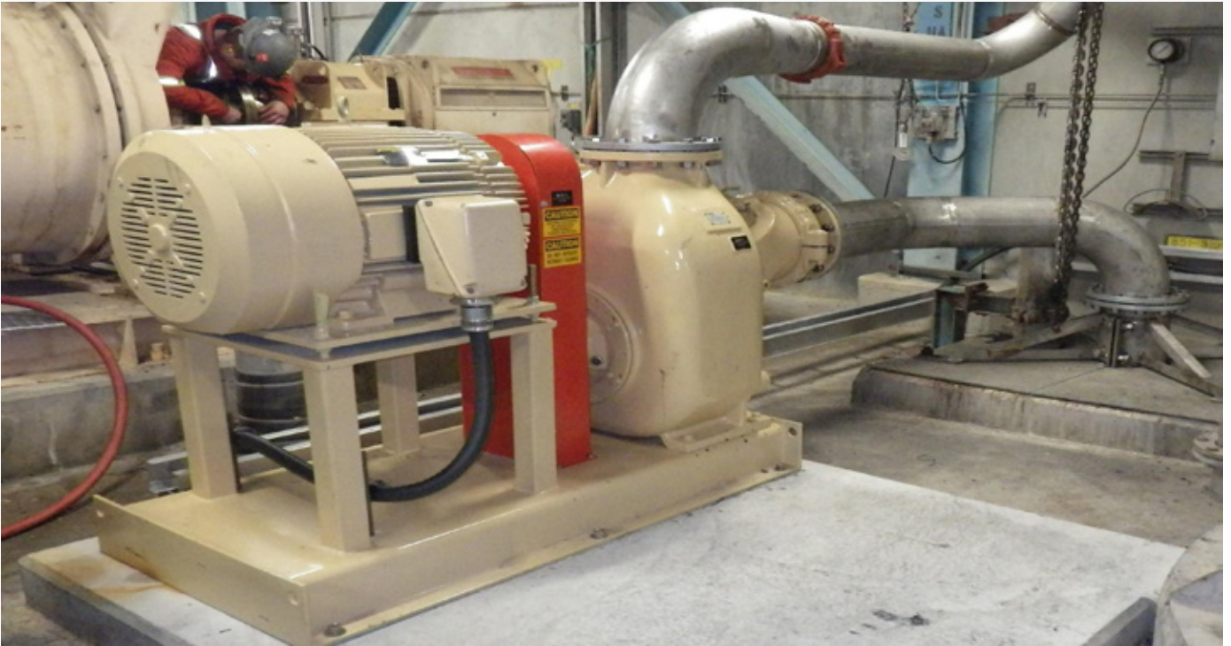
PULP AND PAPER TRANSFER PUMPS Shown TFCC-10 installed at a multinational paper mill in Wisconsin. Belt driven model shown.
